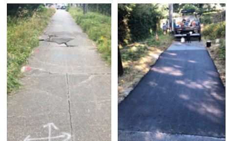
Before (left) and after (right) improvements on the 23rd Ave SW walking/rolling pathway
